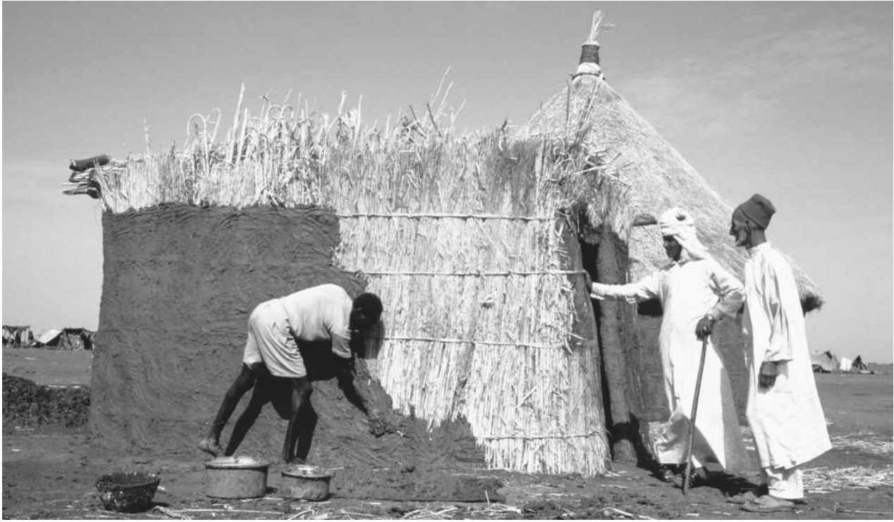
A Rasheida resident employs a worker to mud-plaster his house. These mud structures are common in the northern region of the Sudan.
